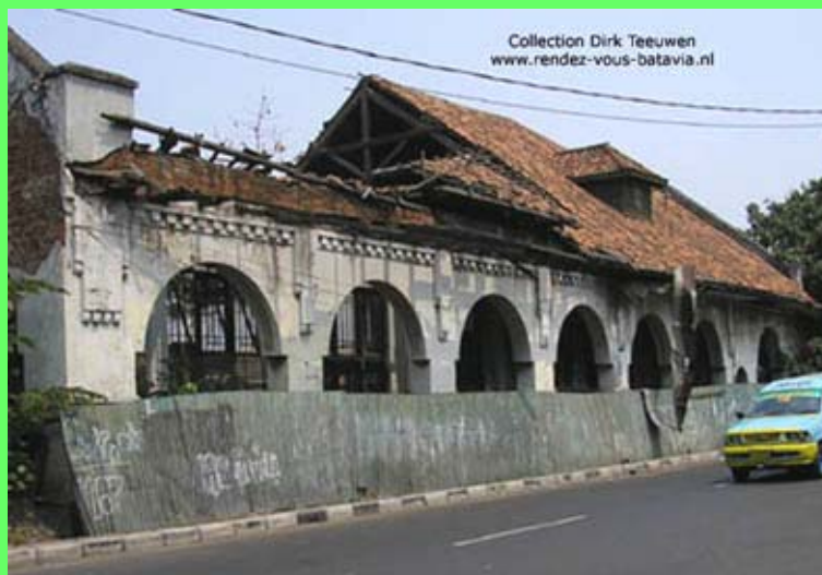
4.2 This is all there is left from the “dispens”, food storehouse and food shop, of the former V.O.C.-castle (V.O.C. means Dutch East India Company), demolished in 1810.
