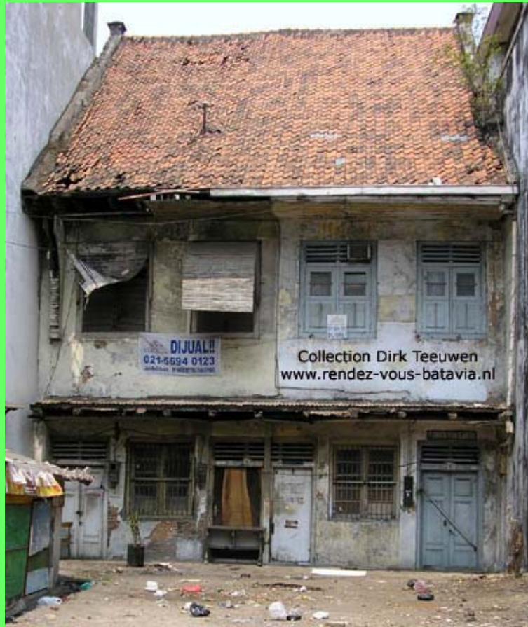
4.1 A Dutch house from about 1750 in terrible state along Rua Malaka, to the west of Kali Besar.
